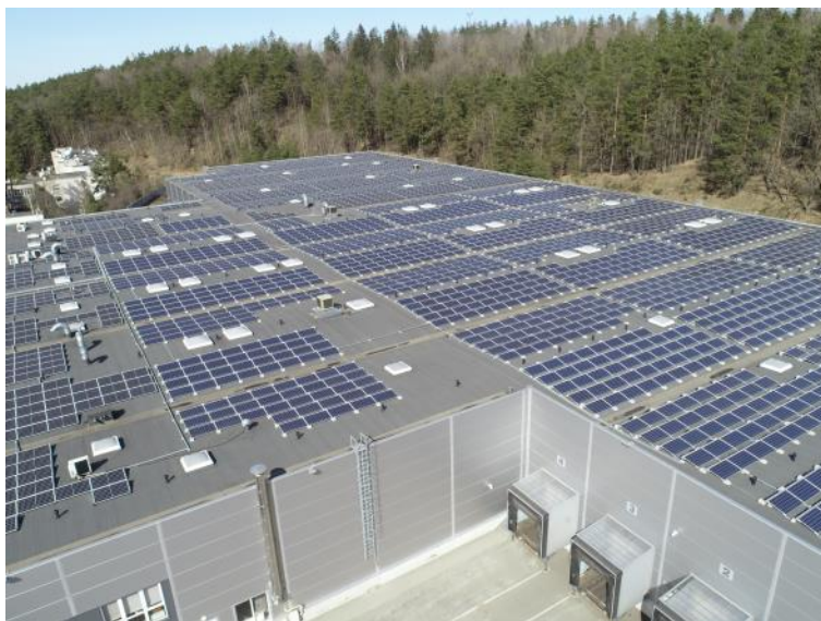
Aerial photo: The solar power plant on the roof of HPP Baltic Sorting Centre in Vilnius.
